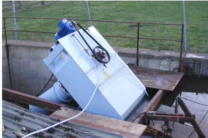
10kW siphonic propeller turbine at Borrowash Mill
